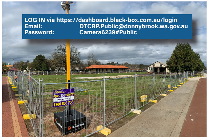
The site of the Donnybrook Town Centre Revitalisation is now fenced off and ready for construction. The public can view updates via Blackbox.
