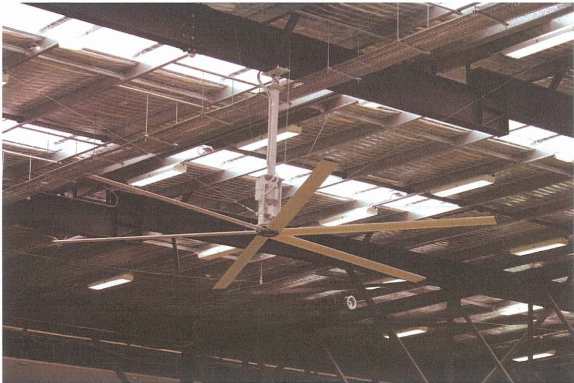
Photograph No. 1 Roof Mounted Fan
