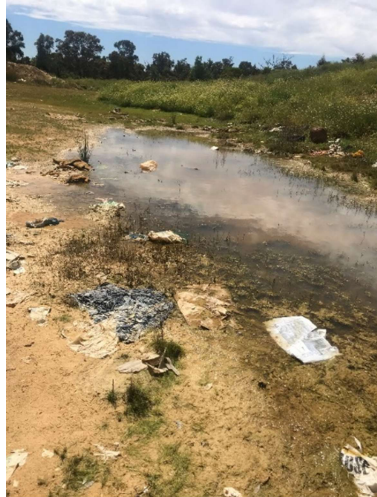
Photograph 11: Ponding stormwater at the northwest corner of the landfill.
